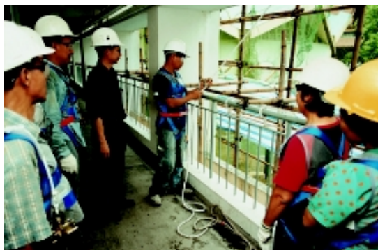
The foreman is teaching workers how to use the safety belt correctly
