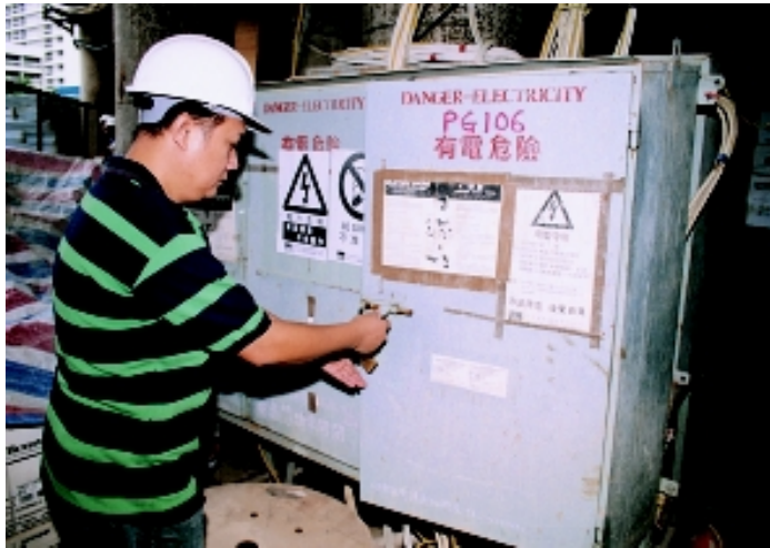
The foreman is checking the switch box
