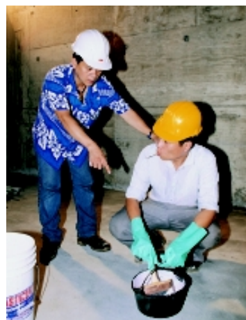
The foreman is correcting the at risk act of the worker
