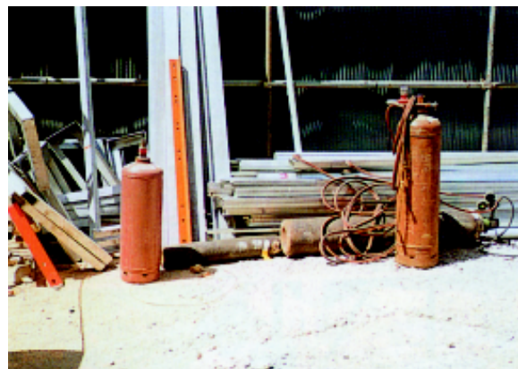
Mixed storage of empty & filled gas cylinders
