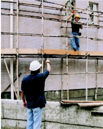
The foreman is directing workers to abide by the safety operation procedure
