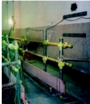
All the passageways are cleaned up; trash and waste have been properly removed
