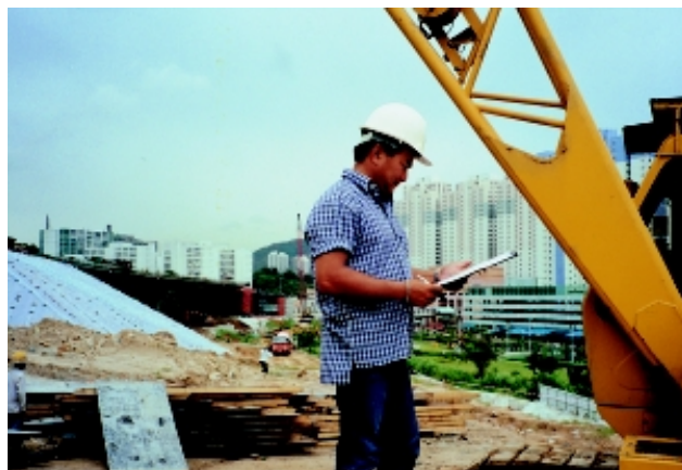
A competent person is carrying out the monthly inspection on the mobile crane as required by the contractor
